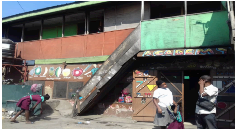
State of the Kayayeei Children's School before refurbishment
